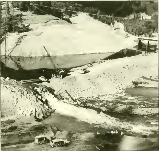
Cofferdam impoundment near Trinity Dam marking the beginning of flow regulation in 1958. Trinity and Lewiston dams were completed in 1964.
